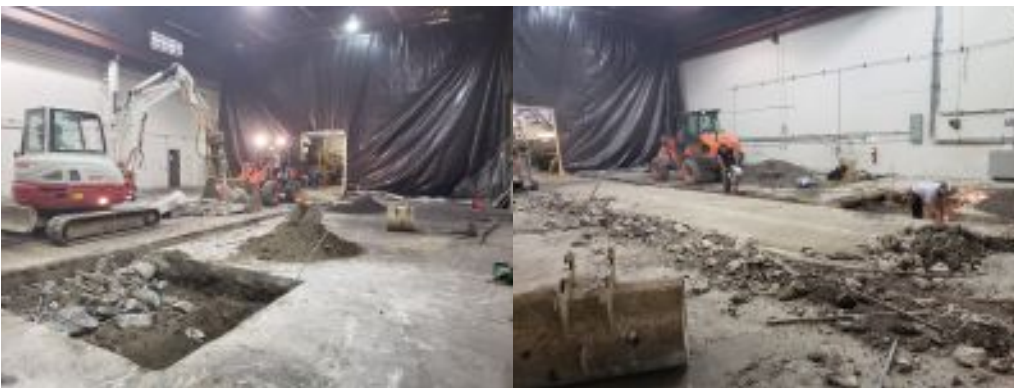
Pictures of construction work being done to prepare the area for the Gen3 PUREVAP™ pilot plant. All images © PyroGenesis
